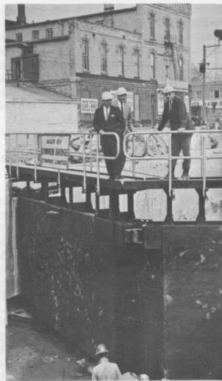
Three members of the canals division viewing the progress of construction from the rear lockgate last May. Left to right: Dave Bennett, superintending engineer, Trent Canal (Mr. Bennett was transferred to headquarters this month); Herman Granx, headquarters engineer; and Keith Oglesbey, the author.
