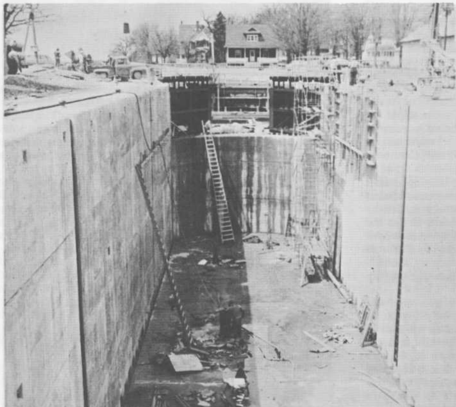
Construction of the lock itself got underway in October, 1962. This picture was taken in April only three months before it was filled with water and locking through boats of many shapes and sizes.
