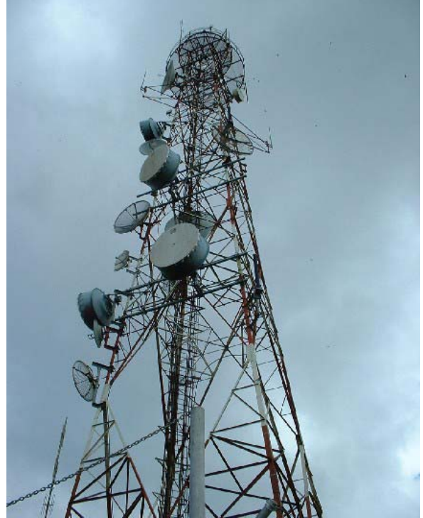
The Instituto Costarricense de Electricidad (ICE, pronounced "EE-SAY") tower #1 at Vista el Mar. There are two ICE towers located at this site.
