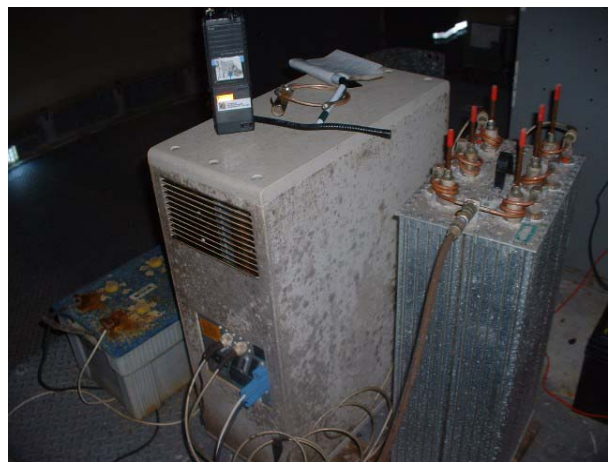
An abandoned Motorola MSR2000 VHF repeater and a Sinclair Q2330E duplexer — both reduced to "rust balls" and no longer serviceable after 10 years in the Azul environment.
